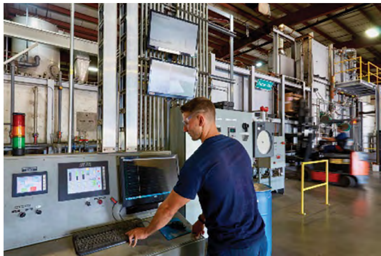
Figure 2: Lower temperature thermal reduction in combination with advanced environmental controls greatly reduces emissions. (Source: TRu3Tec system, Gannon & Scott Inc.)
